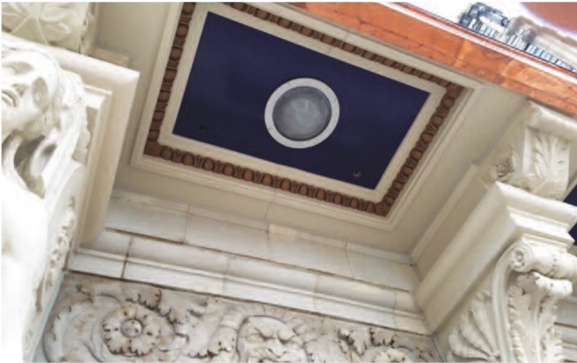
The entire east cornice of the Book Building was removed and replicated, including installing new support steel, replicating the original ornamentation in glass fiber reinforced polymer, and replacing the cornice's deteriorated copper sections with newly fabricated copper.
